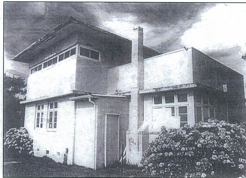
PHOTO 9 (Top): The Red Bluff battery observation post in a very dilapidated condition (1990)
