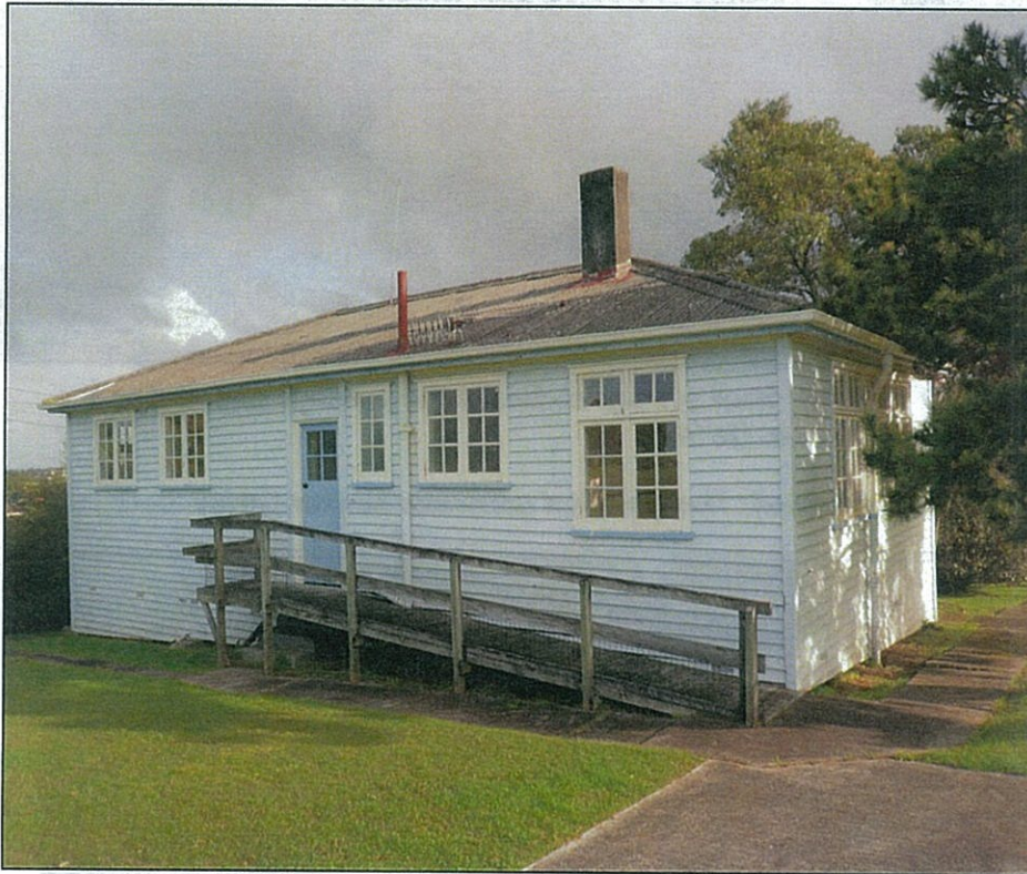
PHOTO 14: The former Red Bluff recreation hut (139 Beach Rd., Castor Bay) currently owned by the Housing N.Z. Corporation (2010)
